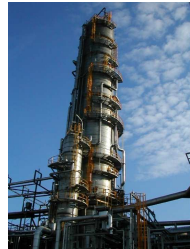
Crude Oil Unit
